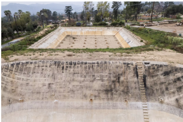
This image shows two water reservoirs that were dry after being damaged in the Eaton Fire in Altadena. Photo credit: Myung J. Chun.
